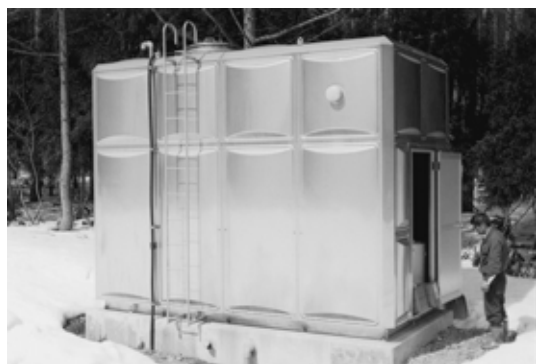
Fig. 4 Hot water tank and its shield. Small ventilating duct and manhole are visible on the roof.
